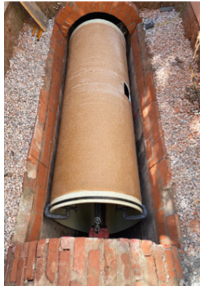
GRP segments are treated with bonded graded aggregate material to enhance adhesion to the annular grout
