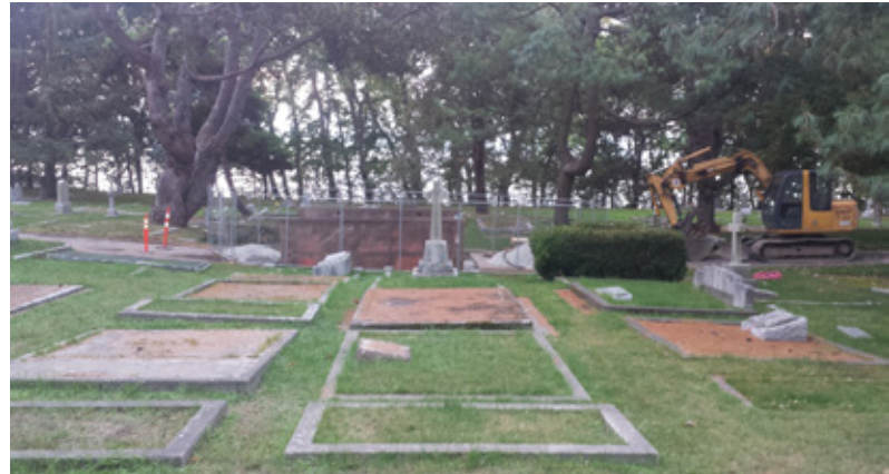
Main service pit was relocated due to utility conflicts with site access was very tight in this predominantly residential neighbourhood
