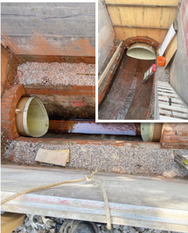
Each 2.4m segment of GRP was carefully pushed together for a watertight joint
