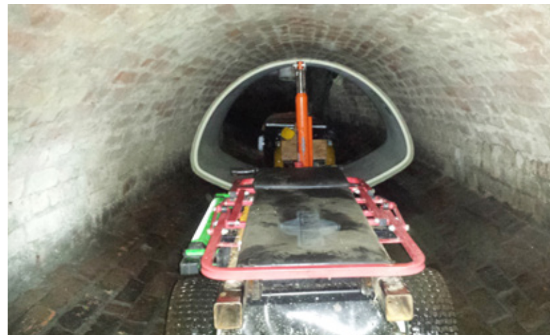
Each GRP segment was maneuvered into place using an electronic motorized cart
