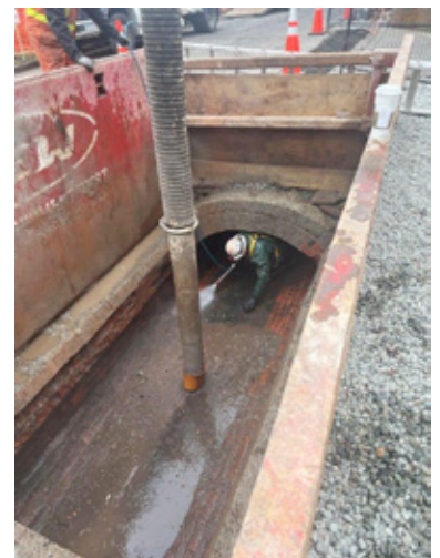
Brick pipes cleaned out using high pressure water, and debris removed by hydrovac
